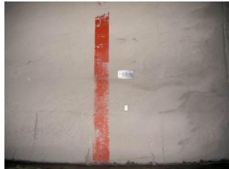
Fig. 16: Wear inside the sediment bypass tunnel (As of January 2016)
