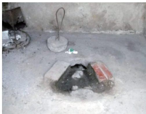
Figure 2. Urine diverting dry toilet at the Trai hamlet study site. (Taken by the author)
