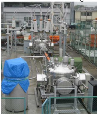
Figure 2. 15m long cable verification system @SEI Feb. 2013[2]
