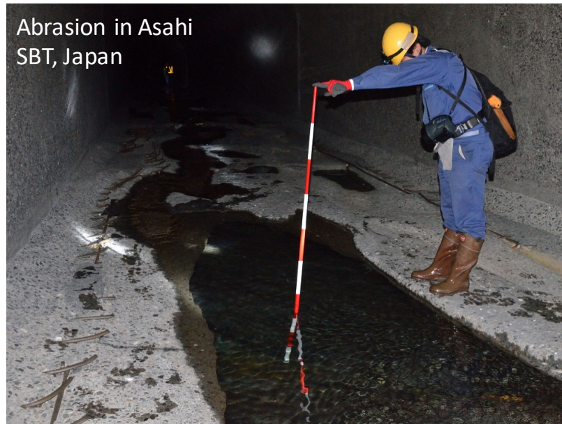
Fig. 2.4 Invert damages at Asahi dam SBT in 2011.
