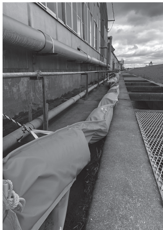
Figure 5. Permanent oil boom implemented in the south side of plant premises, in the closest area to Rokkaku river embankment.
