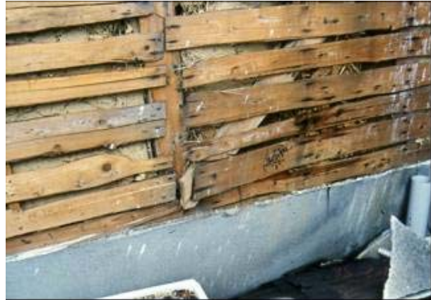
Fig.5 Poor connection between brace and sill or column observed in the 1955 Great Hyogoken-nanbu earthquake.
