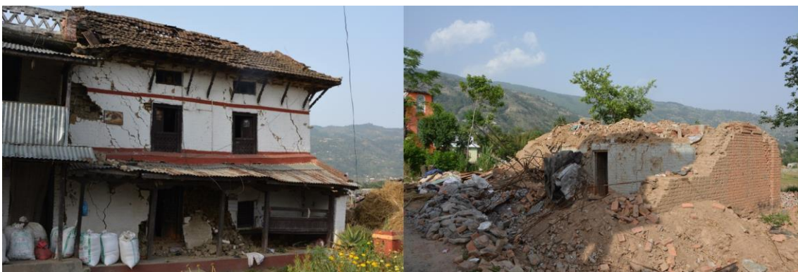
Figure 7. Earthquake damages in Aalapot
