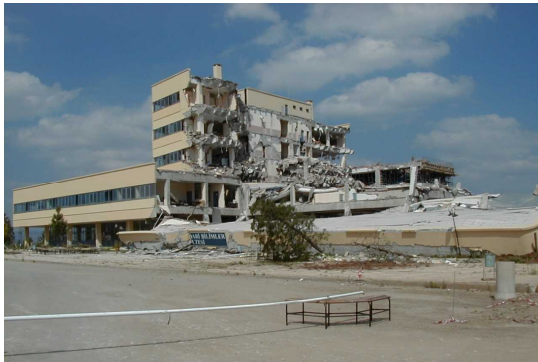
Photo 5. Damaged building of the Kocaeli University under construction of new campus in the Kosekoy region.
