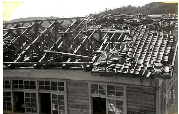
Photo 1. Damage to clay tile roof of low-rise timber building caused by strong wind during typhoon Vera (1959) from DPRI-KU archive.
