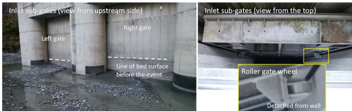
Fig. 3 Disabled SBT gates of Koshiu after the typhoon.
