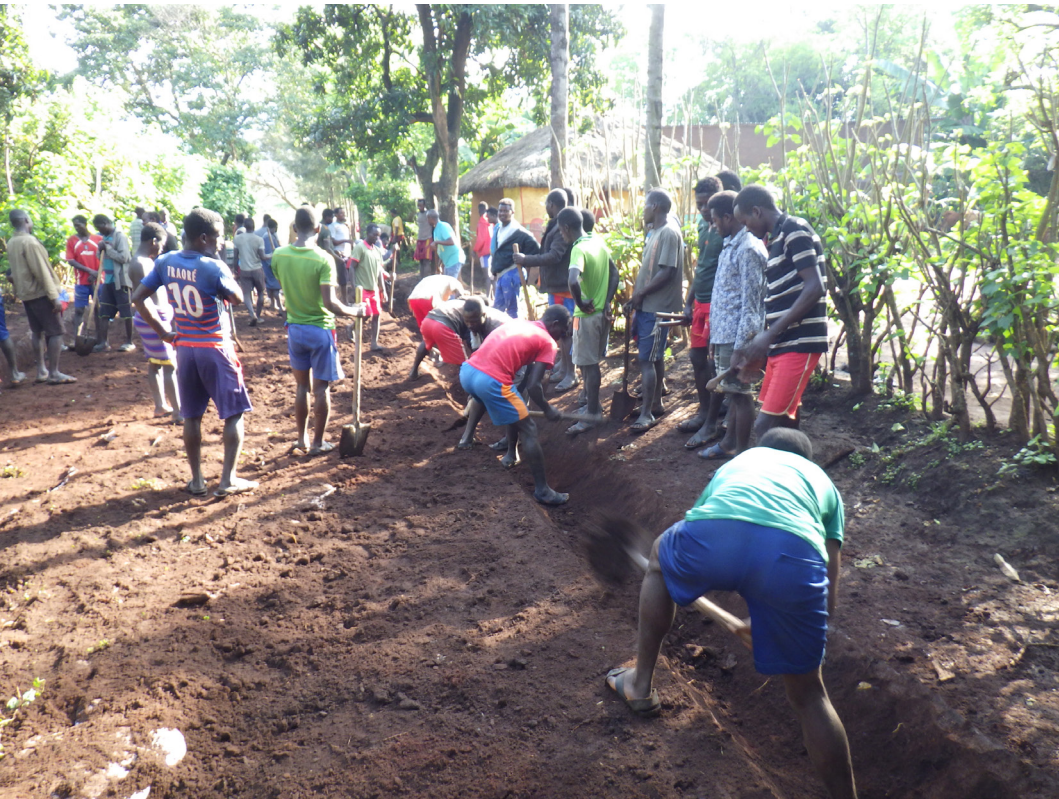
2. Villagers Forming the Gutters for Drainage. They Excavated by Turns. Jinka. December 2019
