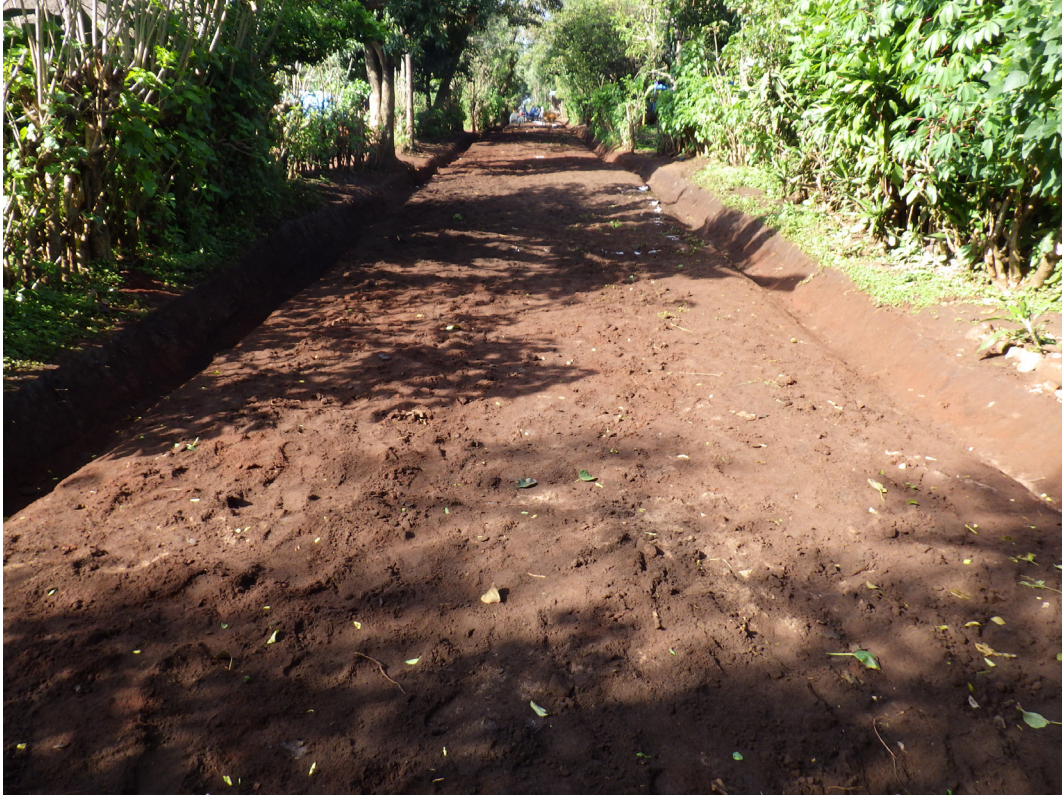
3. Leveled Path and Formed Drainage. Villagers Did It without Heavy Construction Equipment. Jinka. December 2019
