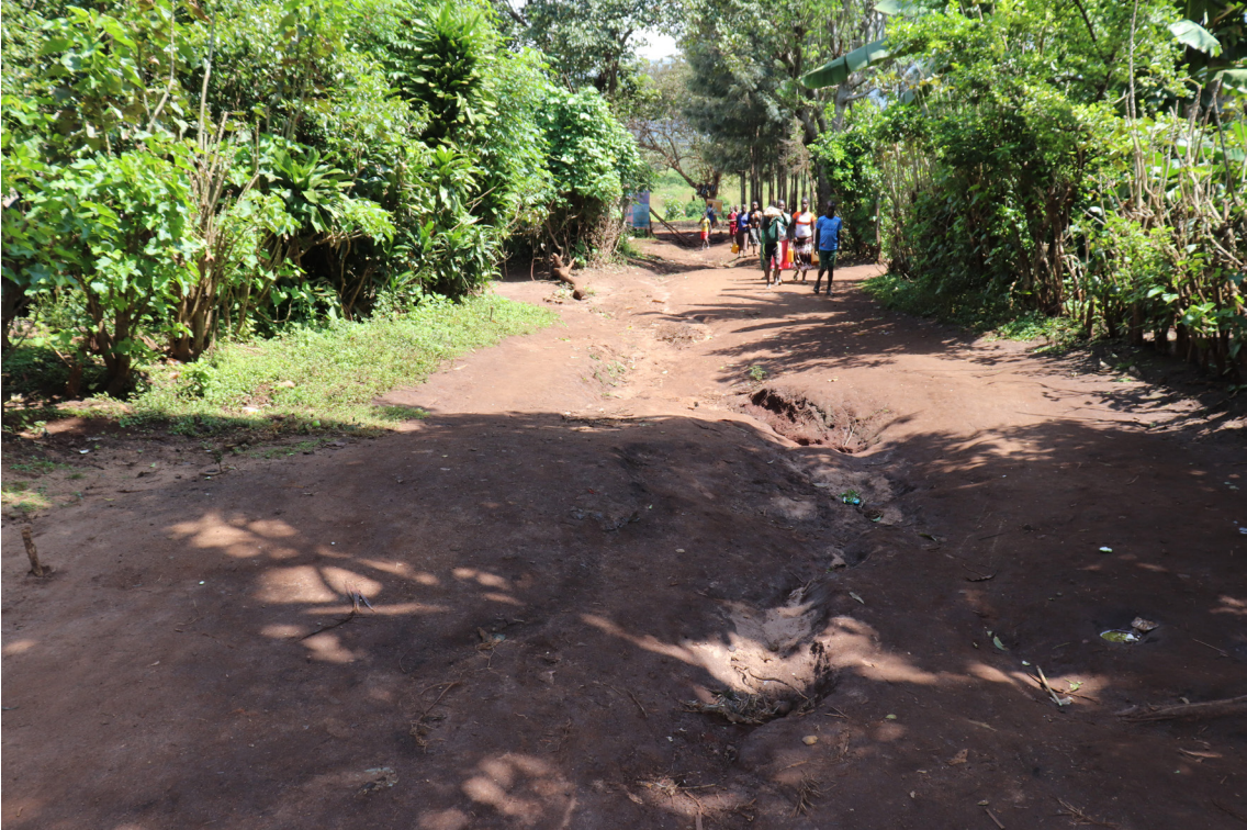
1. Deep Gullies in the Middle of the Path in Front of the Gate of the Primary School Before the Rehabilitation. Jinka. November 2019
