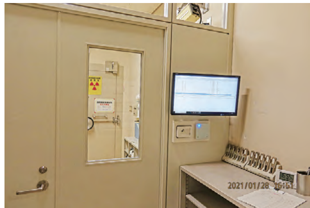
Figure 2. Renewed Entrance and Exit Management System.
