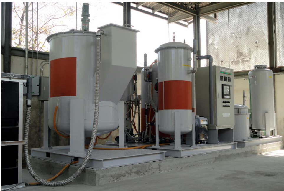
Figure A.2. Biogas plant installed in NakhonNayok Province.
