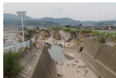
高馬川の堤防決壊箇所(2018 年倉敷市真備町) Dyke breaching of Takama River (Mabi-cho Kurashiki, 2018)
