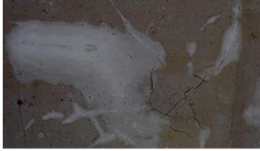
図4 Example of crack
