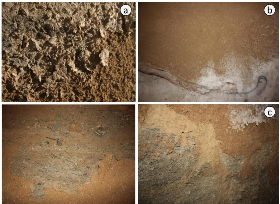
Figure 4.8. Mural deterioration. a) loss of the paint and plaster layer, b) Detachment c) Scaling process
