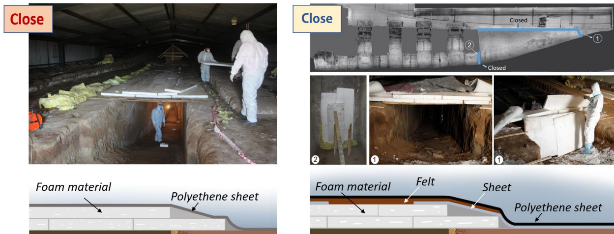
Figure 5.8. Open dromos condition during open and close period. a) Before sealing method, b) After improving the sealing method (1) and closed the first corridor (2)
