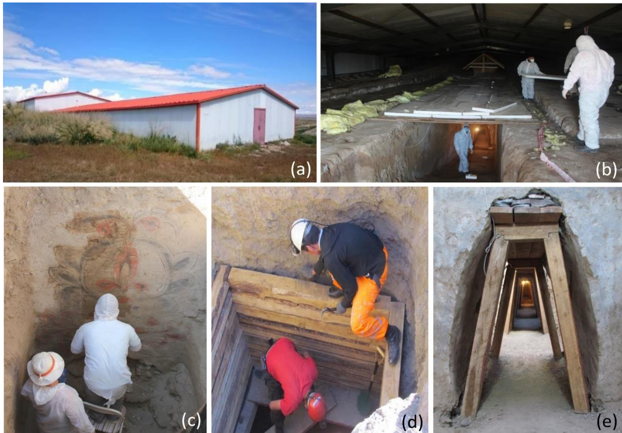
Figure 1.3. Mongolian team carried out protection works for the preservation of the mural paintings in situ. a) Permanent shelter with metal panels, b) Open dromos condition (closure method), c) Consolidation intervention, d), e) Work to prevent the mural painting from collapsing
