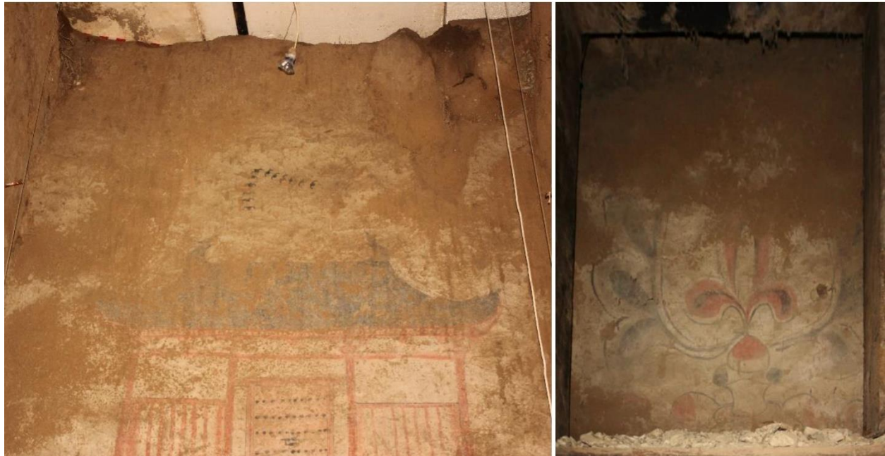
Figure 4.5. Peeling of the mural painting in the upper part of the airshaft
