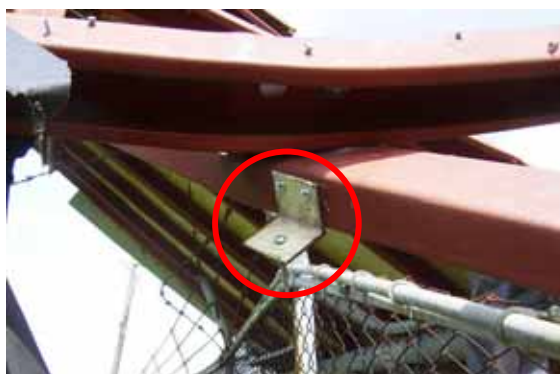
Photo 9 Blown roof and shackle
