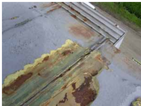
Photo 7 Remained roof surface.
