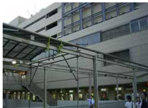
Photo 3 Blown away roofs on a pedestrian bridge.
