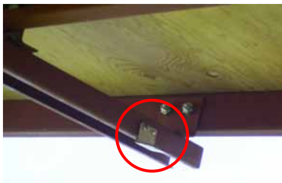
Photo 8 Blown roof and shackle
