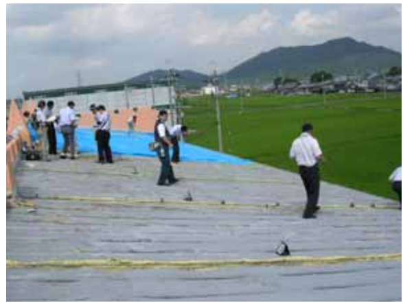
Photo 6 Inspection by police officers on the damaged roof.
