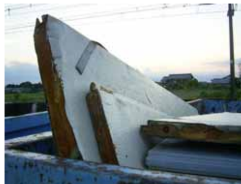
Photo 2 Scattered construction materials.
