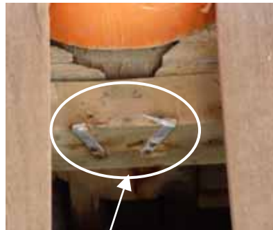
d. Foot of columns of corridor Metal claws used to hold the floor panel in place
