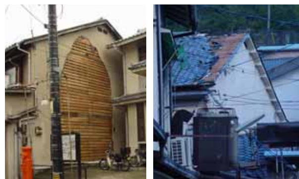
a . A collapsed wall
