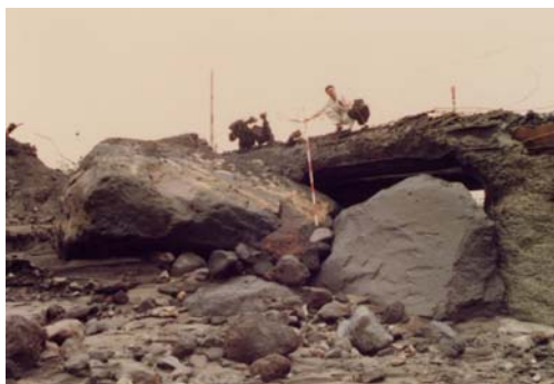
Photo 1 Damages of a bridge at the Nojiri River (July.24, 1982)
