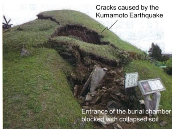
Figure 2. The Kamao Tumulus damaged by the Kumamoto Earthquake (Agency of Cultural Affairs, 2017).
