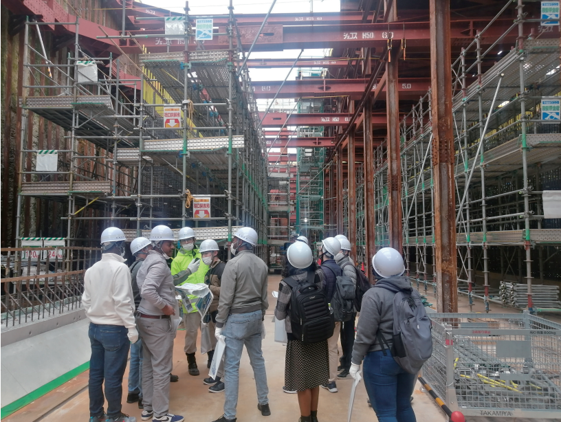
Dec. 5th: The Group Visited the Headquarters of Hanshin Expressway Co., Ltd. at Nakanoshima and Toured the Construction Sites of Open-cut Tunnels at the Osaka Bay Highway West Extension at the Komae Construction Yard.
