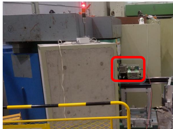
Pic. 1. An overview of the counter installation.
