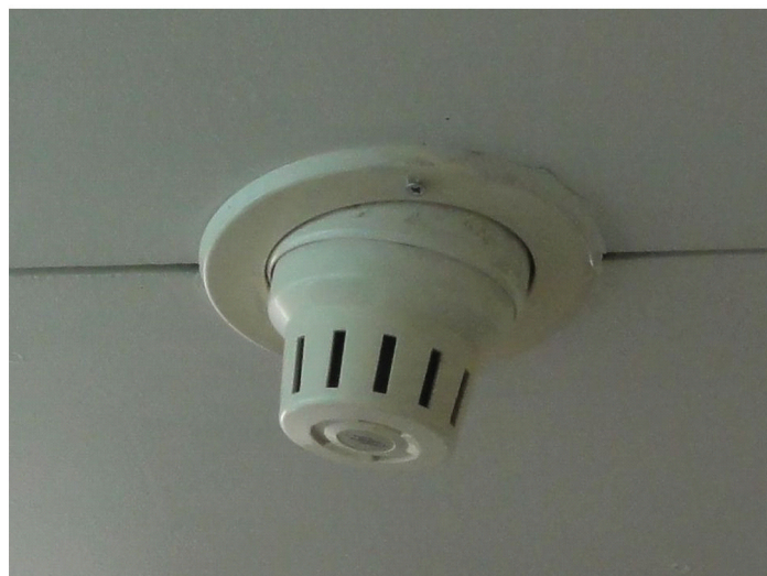
Figure 1. Examples of damage to components of fire protection systems in buildings due to the 2016 Kumamoto earthquake: (A) fire door falling off and (B) fire detector deformation. (The photographs were taken by one of the authors after the earthquake).
