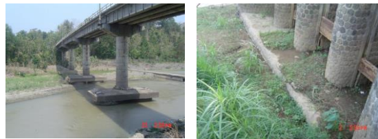
Photo 10 Effects of riverbed degradation by excess sand mining on river structures in Indonesian rivers
