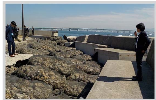
Photo 2 Damaged Kansai International Airport
