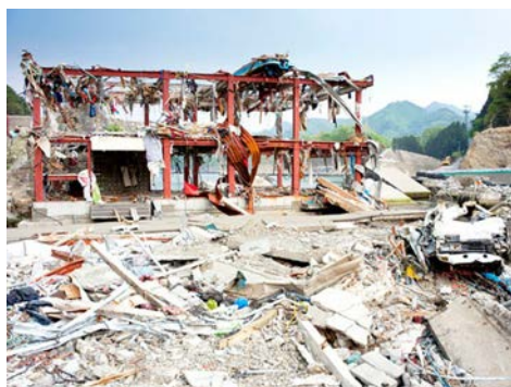
Photo 2 Example of damages from the 2011 East Japan Great Earthquake ( https://weathernews.jp/s/topics/201903/040055/ )
