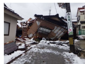
Photo 2-14 Heavily damaged wooden house
