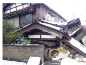
Photo 2-11 Heavily damaged wooden house
