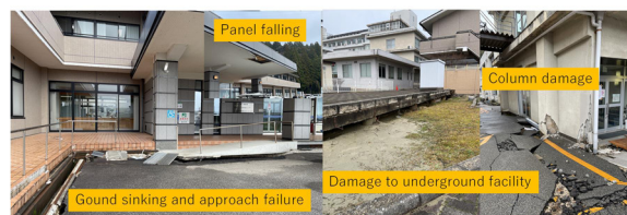
(a) Damage to facilities
