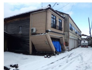
Photo 2-6 Heavily damaged wooden house
