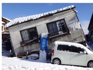
Photo 2-7 Heavily damaged wooden house
