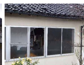
Photo 2-4 Damage to window glass
