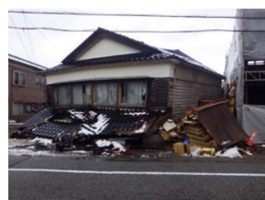
Photo 2-16 Heavily damaged wooden house
