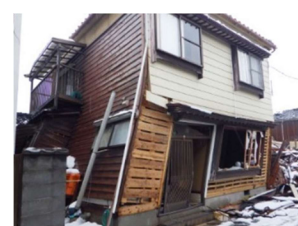
Photo 2-12 Heavily damaged wooden house
