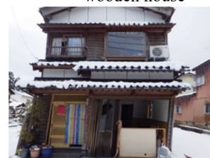
Photo 2-8 Heavily damaged wooden house
