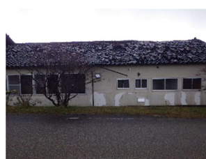
Photo 2-3 Damage to roof tiles
