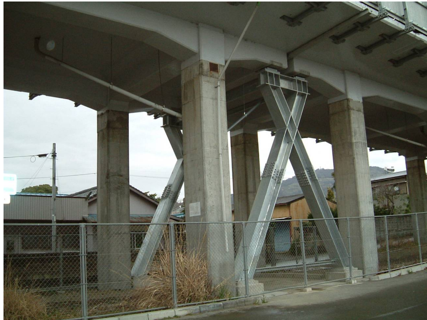
Fig. 5.10: A picture of a reinforced viaduct. This picture is from Hara et al. (2004).
