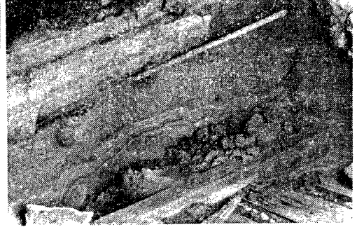
Photo. 7 Scene of the saw dust in layers in the ceiling.
