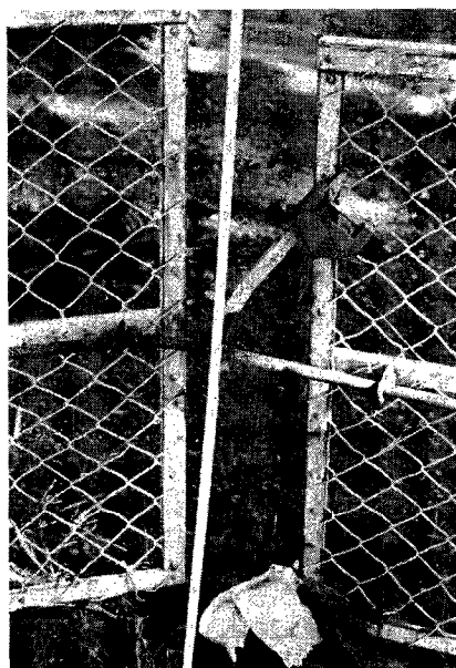
Photo. 7 Bended iron bar of the door of the house.
