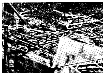
Photo. 4. Roof failure due to uplift: wooden house.
