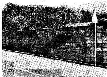
Photo. 15. Failure of concrete block fence.
