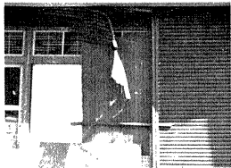
Photo. 25. Damage to the steel shutter in Watomari.
