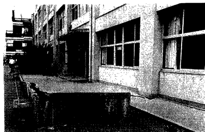
Photo. 2 Damage of slope for carrier cars of school lunch (Tomizuka primary school).
