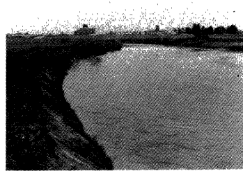
Photo. 3 Bank erosion in the low water course of Katsura River at 1.8 km site, looking upstream (April 10, 1982).
