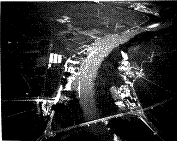
Photo. 3 Bird's-eye view of bank erosion and failure of revetment near Doonura Bridge (3.6 km) looking upstream.
