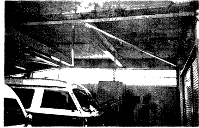
Photo 8 Buckling of horizontal braces
