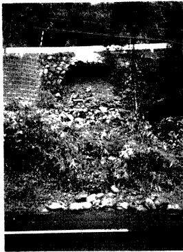
Photo 3 Damage of the edge of road
