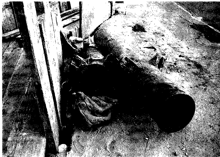
Photo. 32. Failure of a twelve-inch main for AWSS in South-of-Market District (photographed on 11/8/89).
