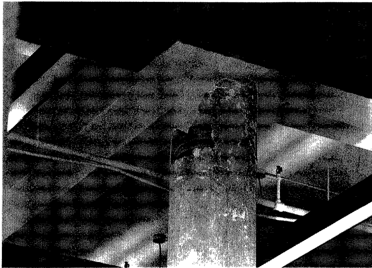
Photo. 15. Bending damage of an RC column.
