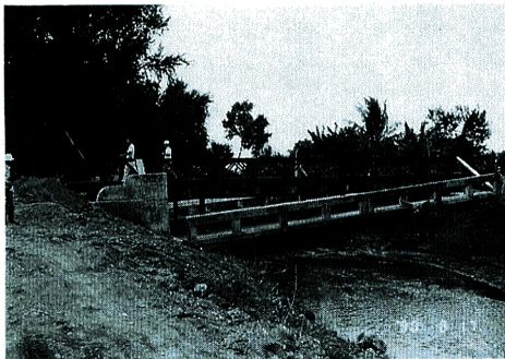
Photo 24 Damage to Maniela bridge.
