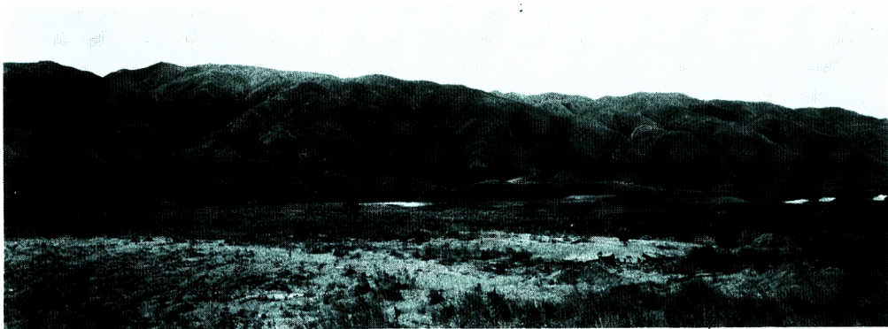
Photo 23 Slope failure toe at Baterya.
