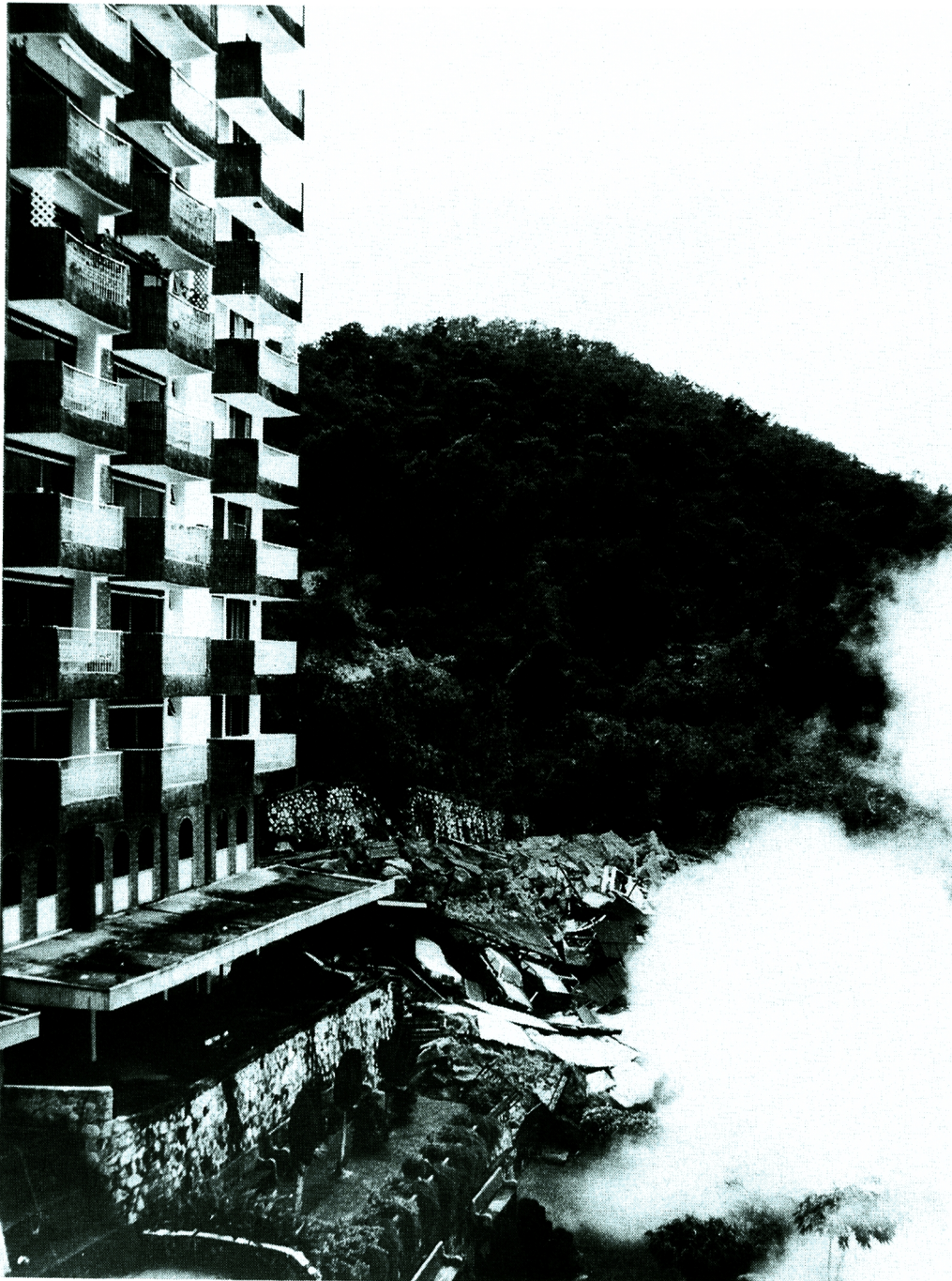
Photo 7 Slid slope and collapsed retaining wall behind the building, 3 minutes after toppling.
