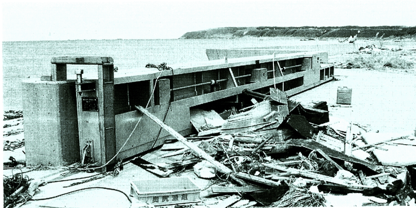
(a) Broken coastal dike
