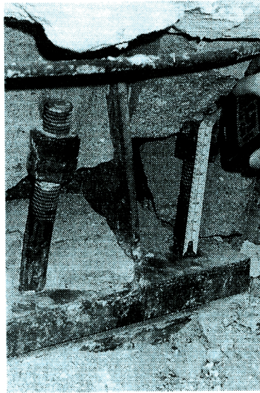
Photo 25 Pull-out of anchor bolts.
