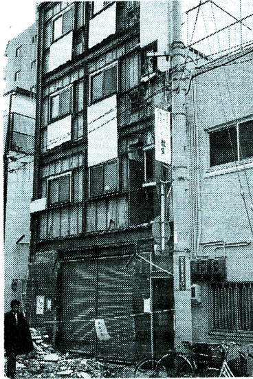
Photo 22 Steel structure with loss of cladding.
