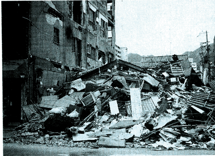
Photo 20 Collapse of 3-story steel structure.
