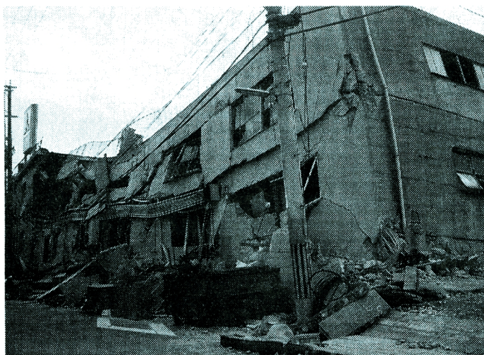
Photo 19 Collapse of a factory building.
