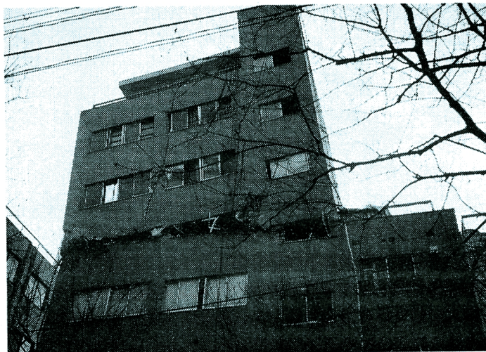
Photo 17 Collapse of upper stories.
