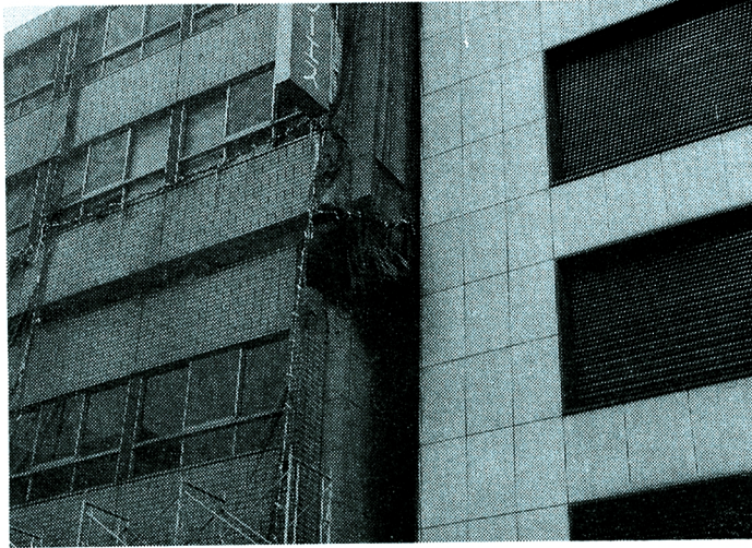
Photo 15 6-story building with a collapsed 4th story.
