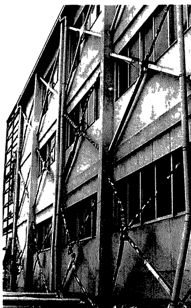
Photo. 3. Damage in a three story steel-frame store: Kyuei Furniture Center.
