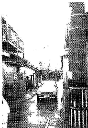
Photo 6. Break of an electric-light pole (Kita, Kushimoto).
