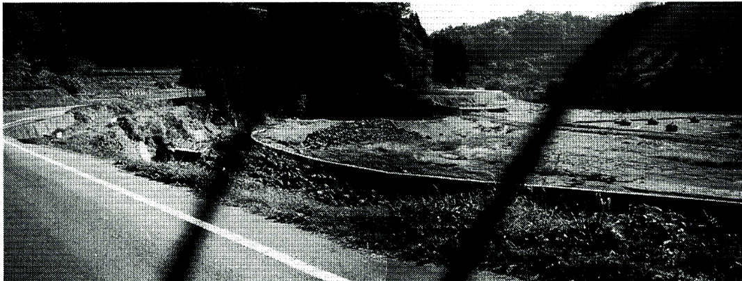
Photo. 3. Channel, floodplain and revetment damage in the Takimizu River.
