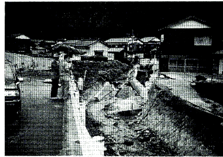
Photo. 3. Failure of revetments in the Satu river.
