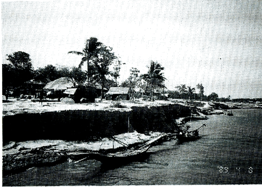
Photo. 1. Bank erosion on right side at No. 9 section.
