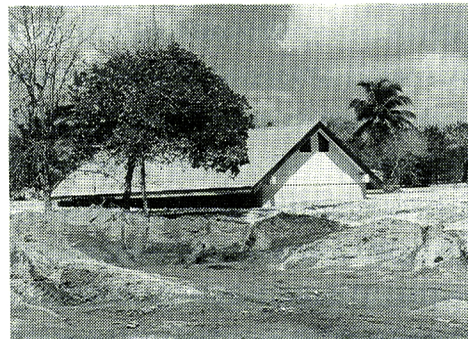
Photo 1. Damaged house by Lahar
