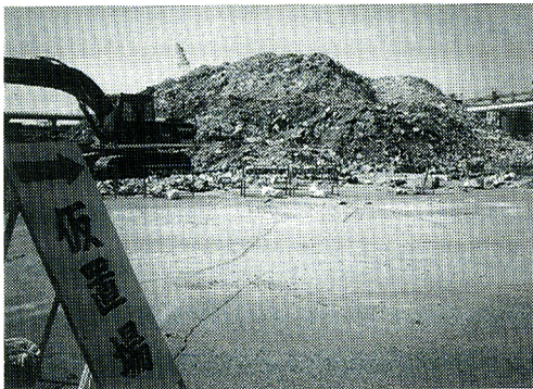
Photo 1. Shipment base (temporary stocking place) of concrete and brick blocks on Kobe's Nadahama.
