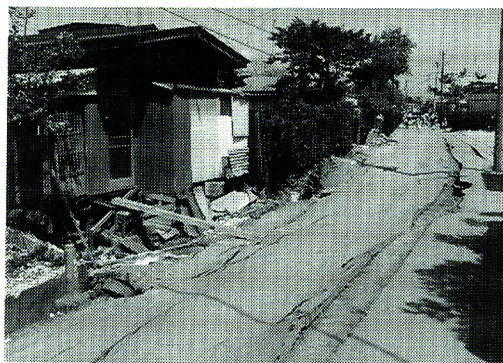
Photo 1. Damage due to liquefaction at Aobamachi in Noshiro.
